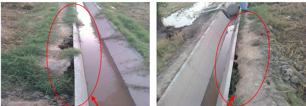
Deteriorated berms due to overflow of water
